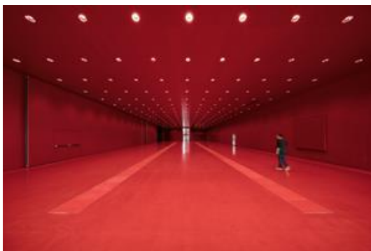
Fig. 5: The round LED recessed downlights PANOS infinity – produced for the Messe Dornbirn in the customised tones of black and red – comprehensively cover every aspect of sophisticated lighting tasks.
