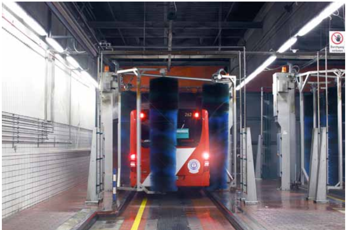
B3 | In the maintenance hangar's carwash facility, too, Scuba luminaires provide sufficient light.
