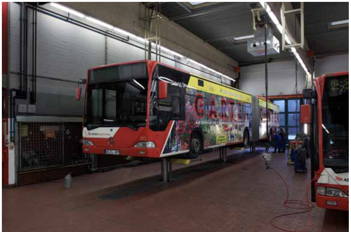
B2 | The Scuba moisture-proof luminaires installed are controlled efficiently via the Luxmate Professional lighting management system.
