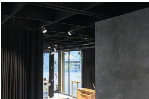
Caption 4: Zumtobel used a specially designed suspension system to install some 160 LED spotlights of the Panos Infinity range in this area. The spotlights are mounted on Tecton trunking.
